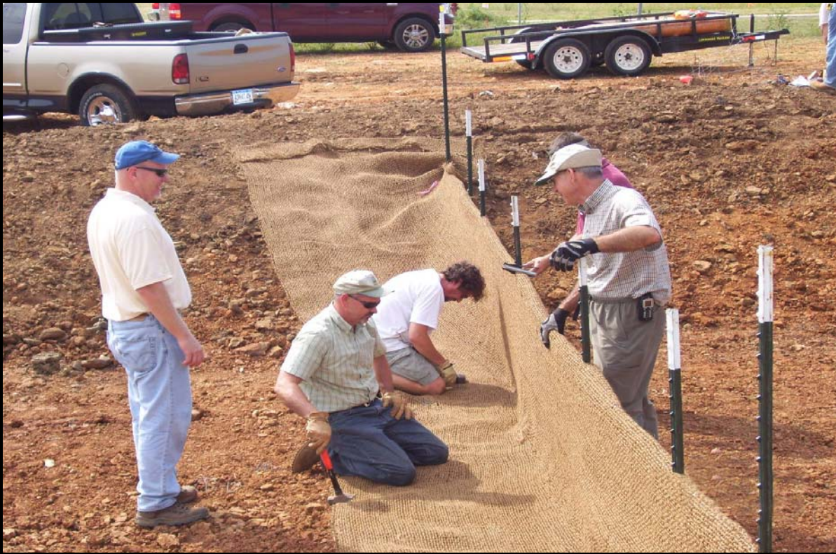
SWCS Members Perry Oakes, Bill Prince and Frank Barnes of Winters Excelsior work to install baffle for sediment basin at field day.
